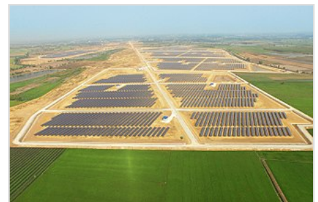
B.Grimm Yanhee solar power plant, Nakhon Pathom, Thailand
